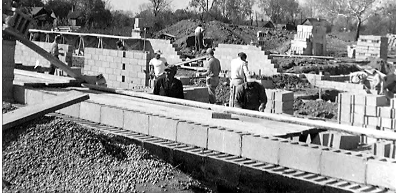
Workers construct Father Thomas Scecina Memorial High School in Indianapolis in this undated photograph. The school will celebrate its 50th anniversary with a Mass on Oct. 24.
