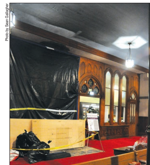
Fire damage is covered and cordoned off on Feb. 28 at the back of St. John the Evangelist Church in Indianapolis.
