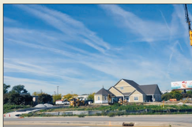
A Women's Care Center is under construction next to the state's largest abortion provider—the Planned Parenthood building on the far left of this photo—on the northwest side of Indianapolis, as seen in this Sept. 26 photo. The new facility will offer pregnancy tests and counseling, ultrasounds, adoption education, classes and other services as an alternative for women considering abortion. The center is set to open in early November, with an official blessing by Archbishop Joseph W. Tobin at 11:30 a.m. on Nov. 18. (Photo by Natalie Hoefler)
