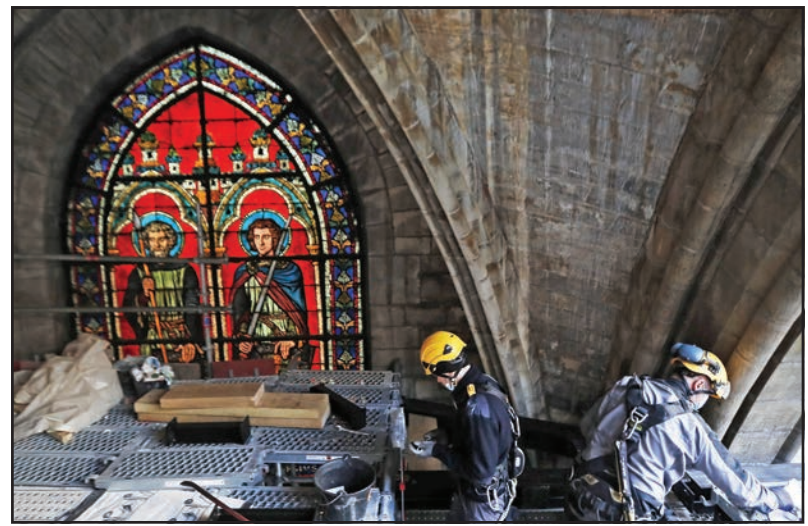
Workers are pictured near a stained-glass window under the vaults at the reconstruction site at the Notre Dame Cathedral in Paris on April 15. (CNS photo/Ian Langsdon, pool via Reuters)
